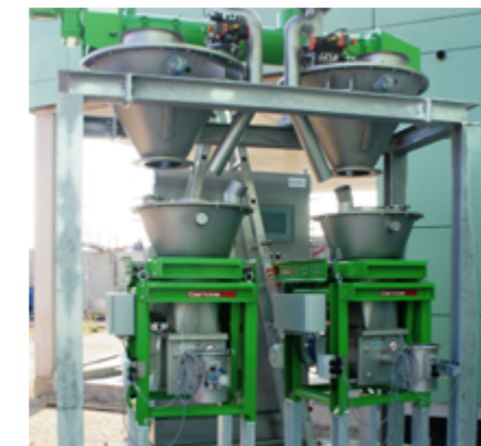
Dosing of activated carbon
